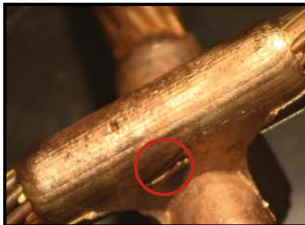
Image 7: Poor connectivity. Visible wire shown in weld.
