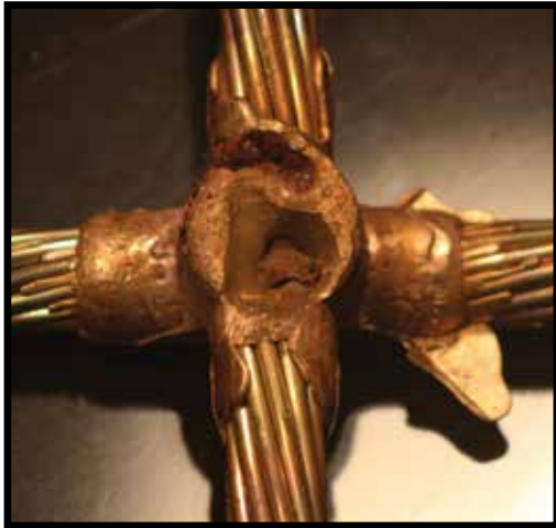
Image 5: Fill too low. Weld cavity was not filled over cable strands.
